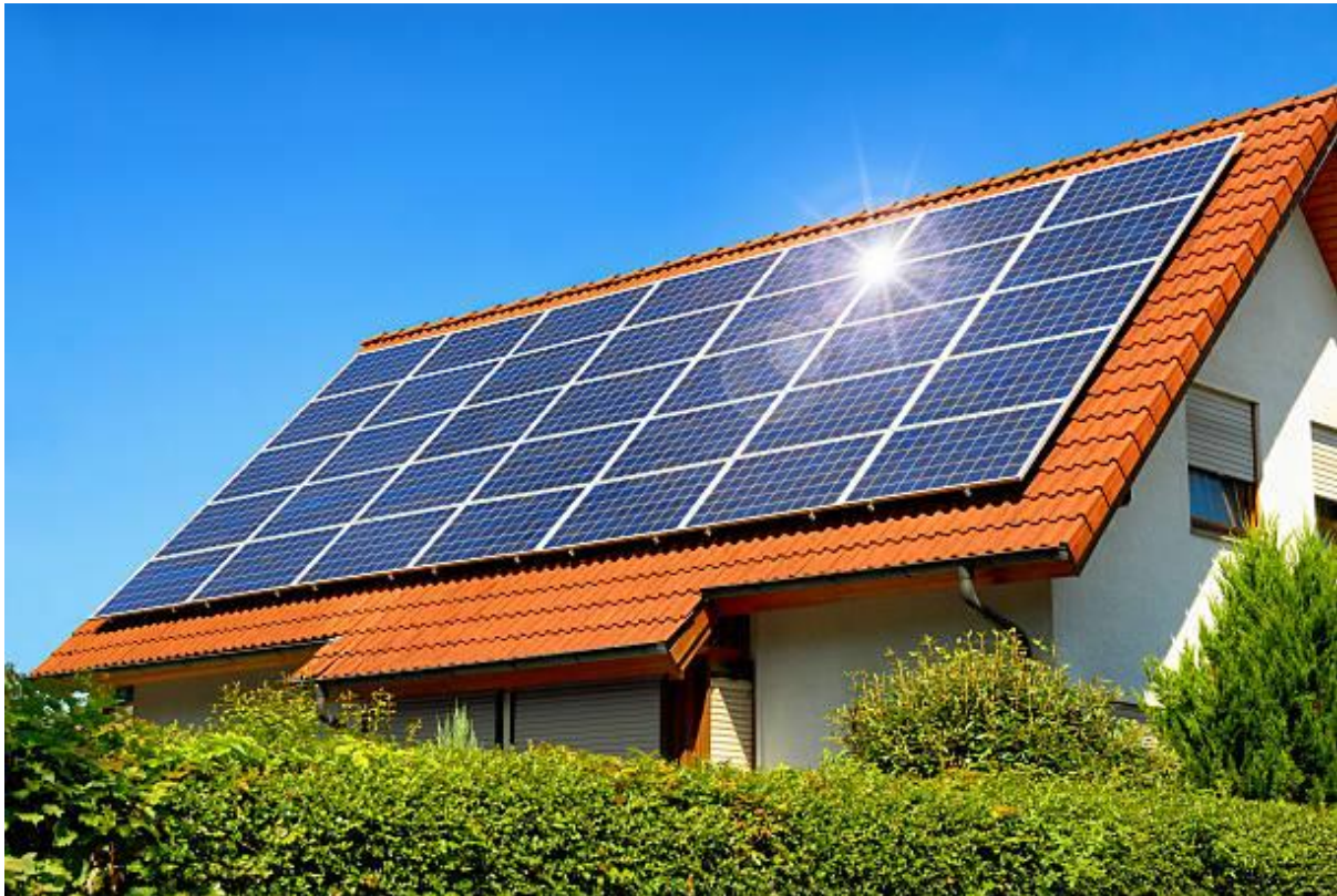
Figure 10.1: Rooftop solar system
